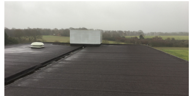
Before: Failed Existing Mineral Felt Roof
