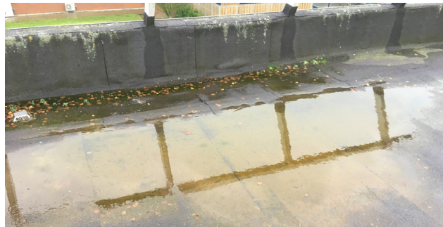
Before: Ponding Issues
