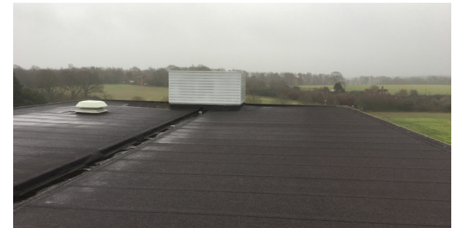
Before: Failed Existing Mineral Felt Roof
