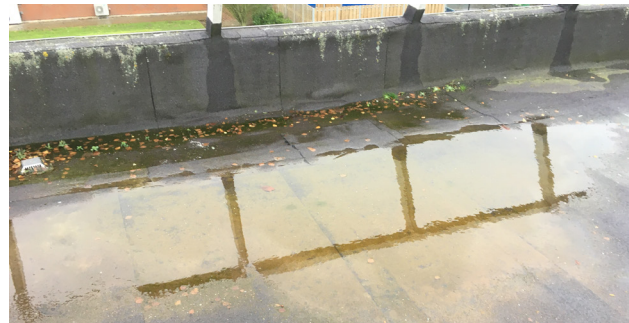
Before: Ponding Issues
