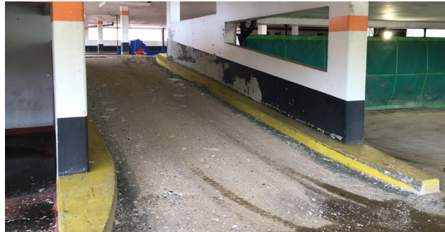
Before: Damaged Internal Ramps
