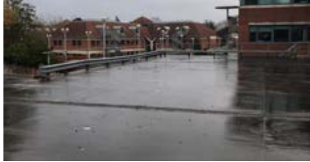
Before: Split & Damaged Asphalt & Drainage
