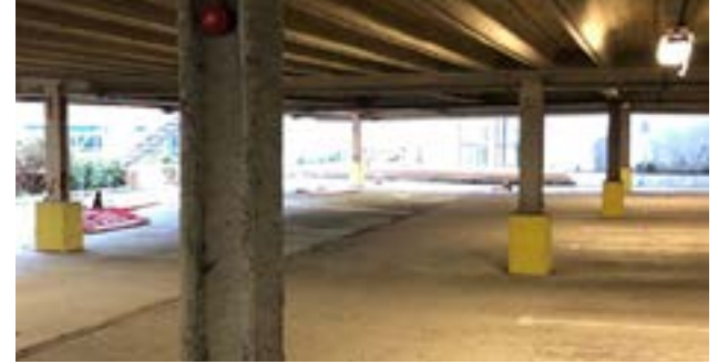
Before: Intumescent Coatings Failed
