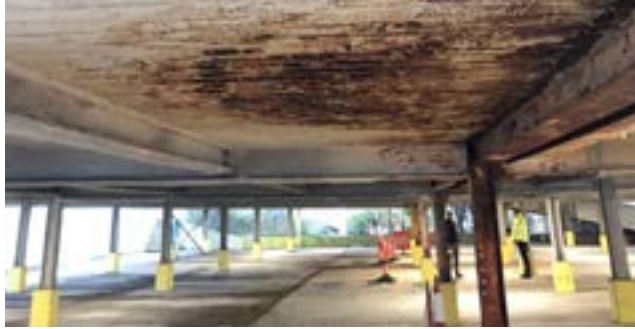
Before: Steel Soffits, Columns & Beams Badly Corroded
