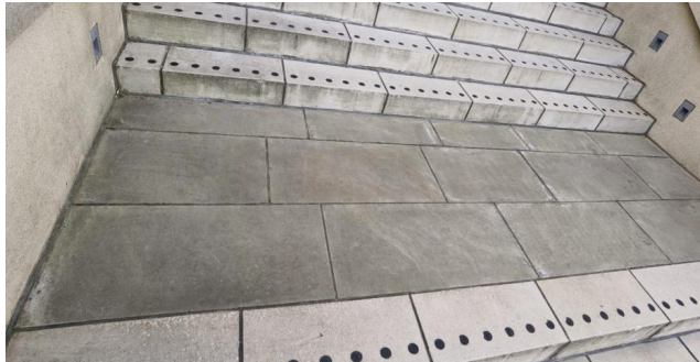
Before: Leaking Entrance Steps
