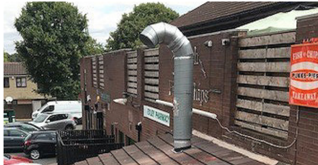
Before: Structurally Unsound Walls
