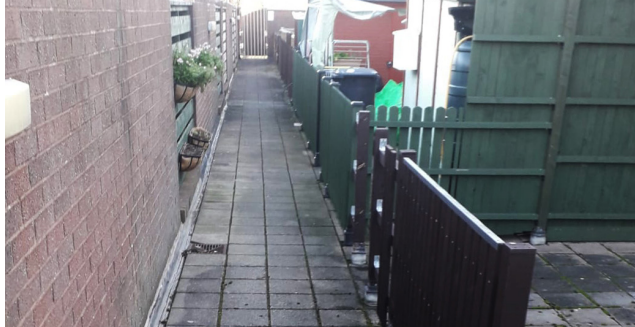
Before: Walkways In Poor Condition
