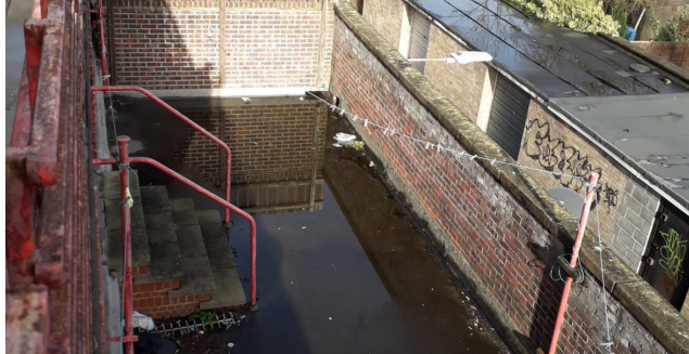
Before: Damaged & Closed-Off Balconies
