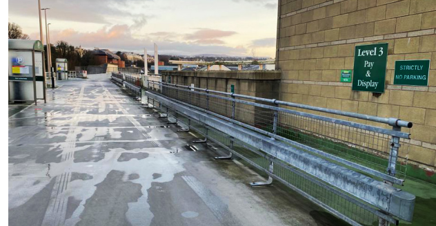
Before: Water Ingress Into Retail & Car Park Levels Below
