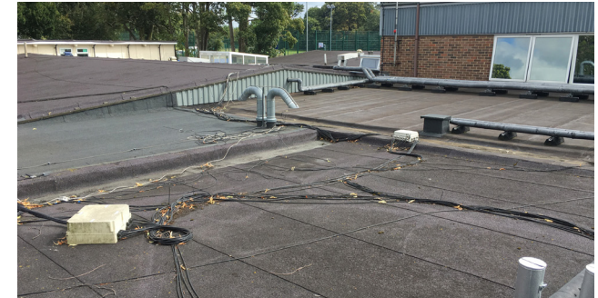
Before: Failed Patch Repairs
