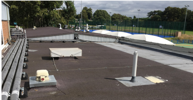
Before: Failed Mineral Felt Waterproofing
