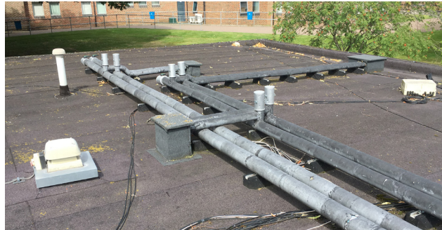
Before: Numerous Cracks in the Mineral Felt
