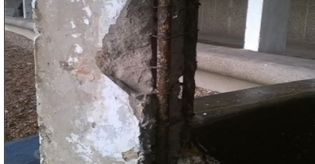
Before: Extensive Concrete Defects
