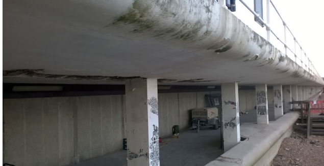
Before: Significant Long-Term Damage
