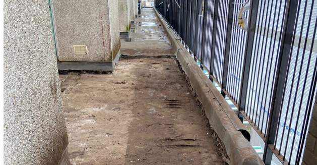
Before: Water Damaged Concrete Slab
