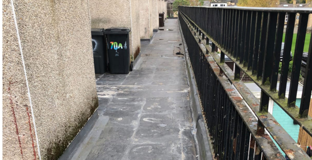
Before: Cracked & Failed Asphalt
