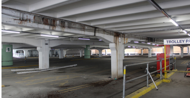
Before: Dark & Unwelcoming Environment With Corroding Steel
