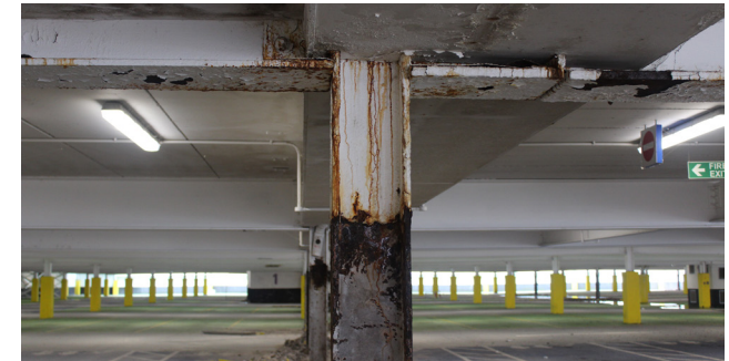
During: Corrosion To The Steels
