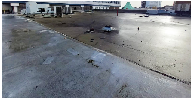
Before: Existing Waterproofing System Damaged
