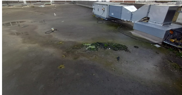
Before: Vegetation Growth to Several Roof Decks
