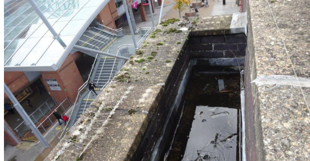
Before: Ponding Water
