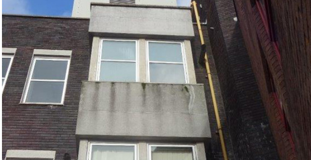
Before: Cracked Facade
