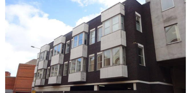
Before: Aged Facade
