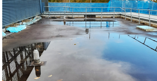
Before: Ponding Issues
