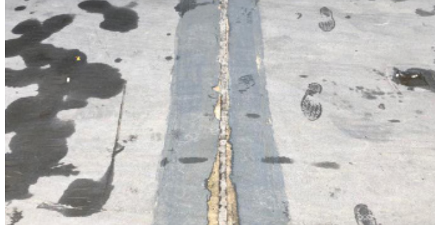
Before: Movement Joints Leaking Into Car Park Below
