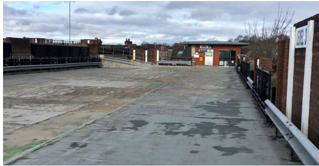
Before: Existing Failed Waterproofing System
