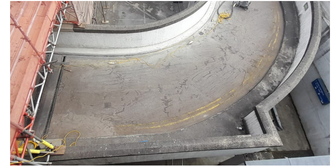
Before: Failed Mechanical Movement Joint
