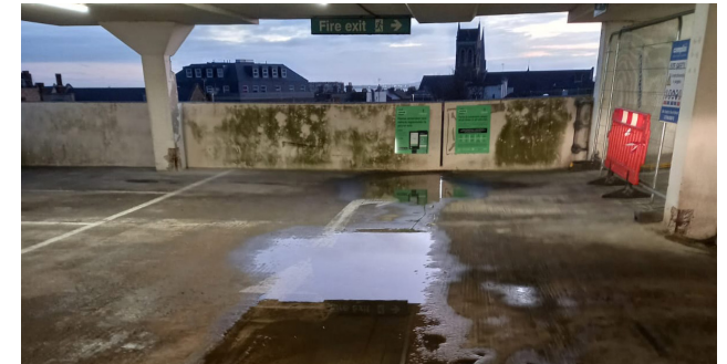
Before: Ponding Water Due To Prevailing Winds
