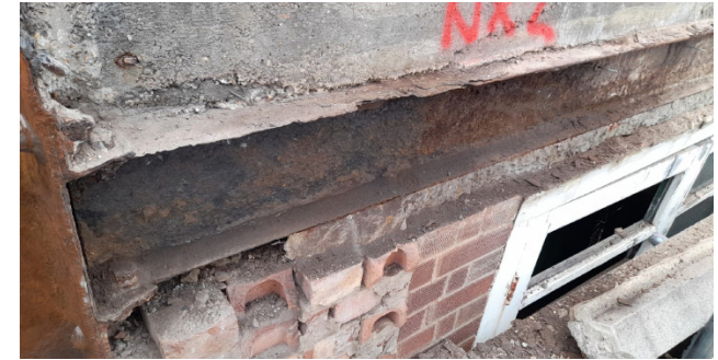
Before: Defective Cills & Building Frame
