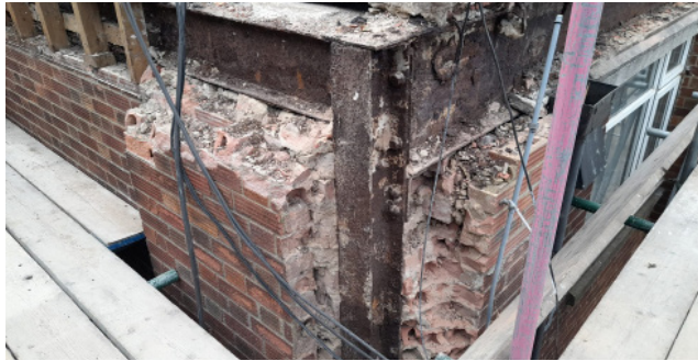
Before: Heavily Corroded Steelwork
