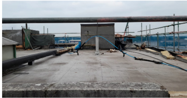
Before: Roof Substrate Allowing Water Ingress
