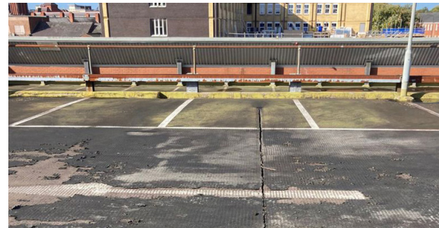
Before: Existing Waterproof Coatings Debonding
