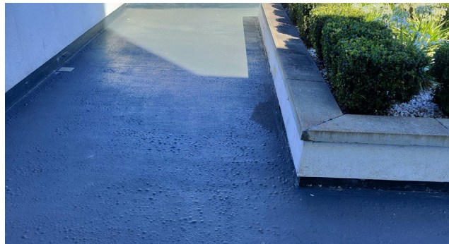
Before: Blisters Caused By Outgassing
