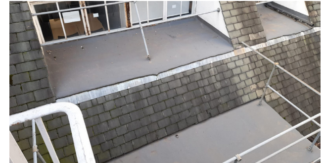
Before: Poor Asphalt Detail At Junction With Lead Flashing
