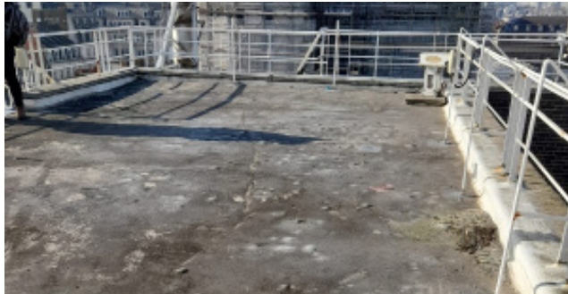
Before: Existing, Failed Waterproofing System
