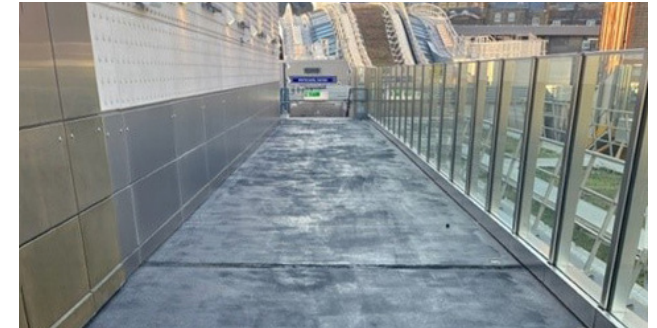
Before: Walkways In Poor Condition
