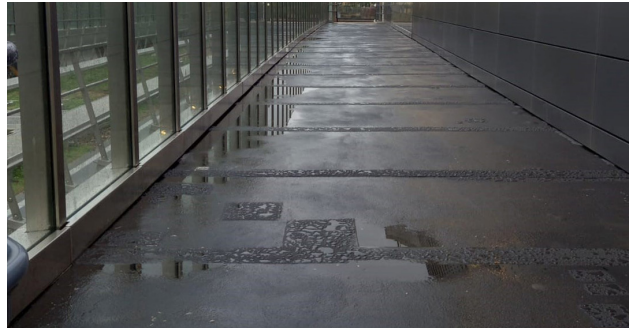
Before: Patch Repairs Previously Undertaken
