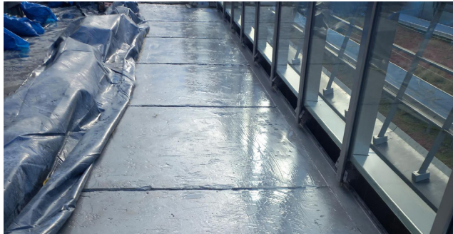
Before: Unsuitable Expansion Joint Size
